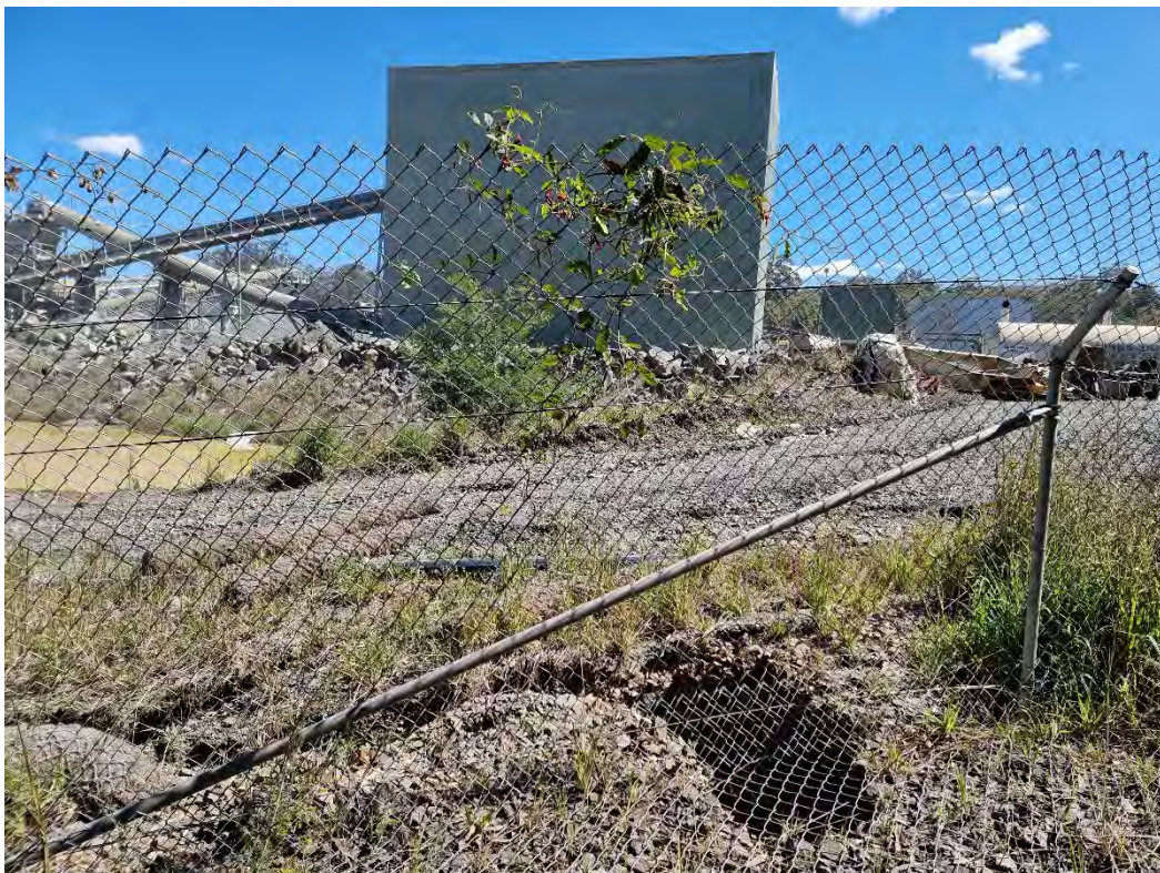
Photo 11: No sediment fencing installed at the time of fence repair (2024) resulting in further erosion (2025).
