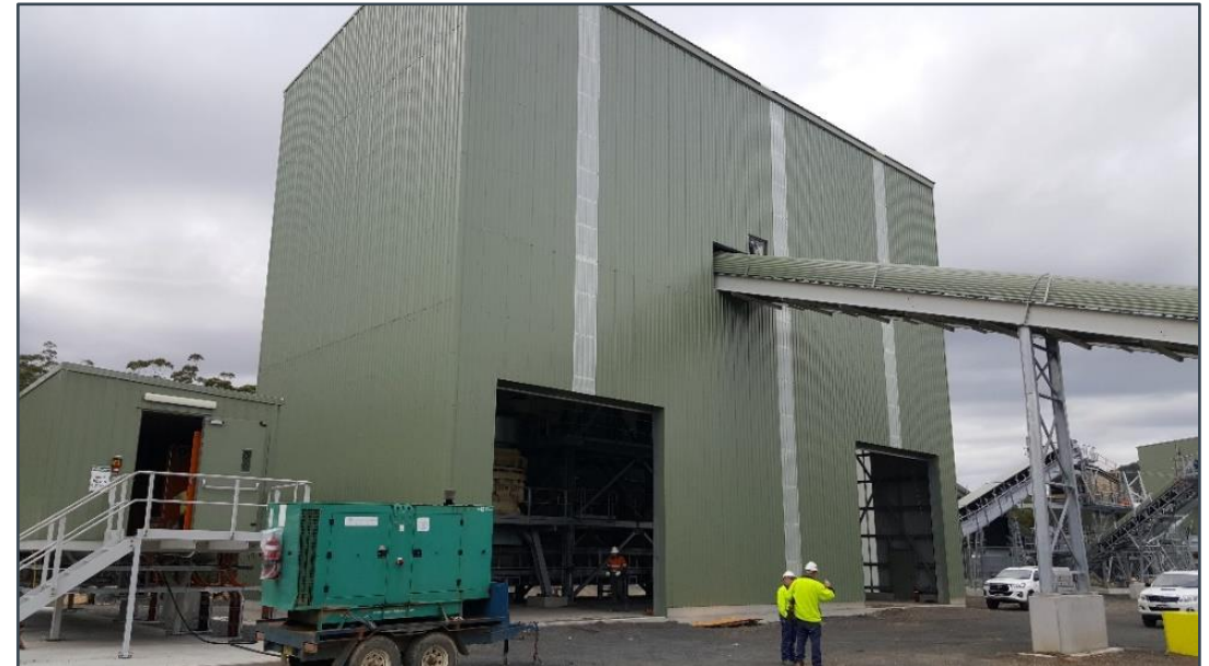
Figure 4: KEQ Secondary (Cone) Crusher Enclosure
