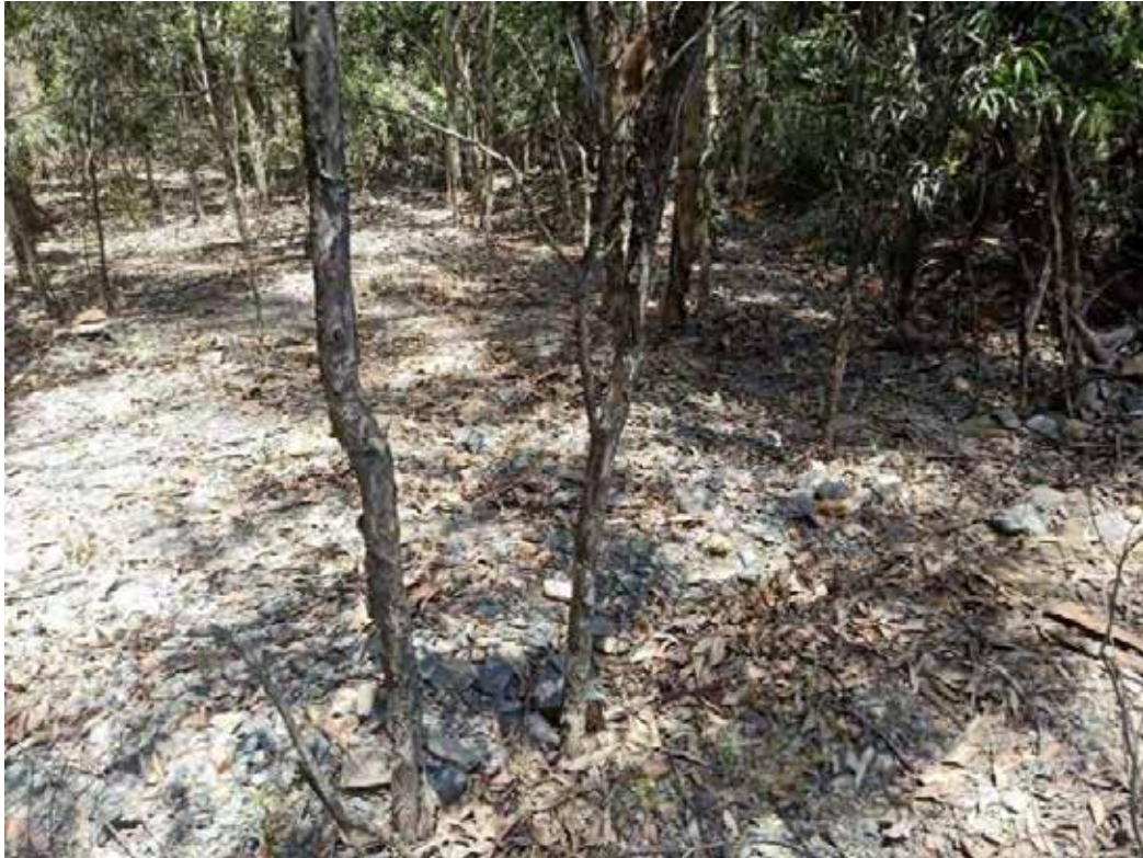
Photo 10: Excavated rock and sediment that has runoff from the eastern boundary of the quarry into the BOA.
