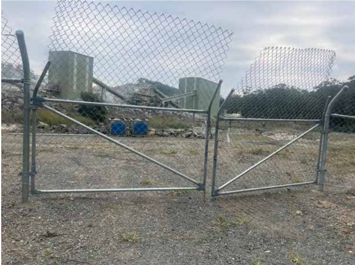
Photo 6: New gate and fencing installed in 2024 along a section of the eastern border of the quarry within Lot 13.
