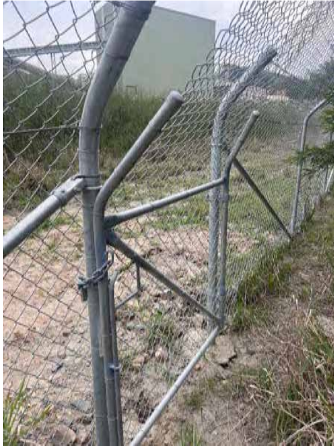
Photo 7: New gate and fencing installed in 2024 along the eastern border of the rock crushing area within Lot 13.
