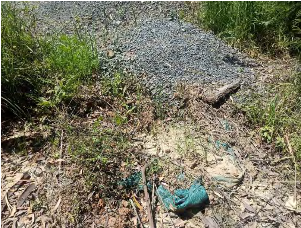
Photo 9: Sediment fencing down and overtopping within Lot 12.
