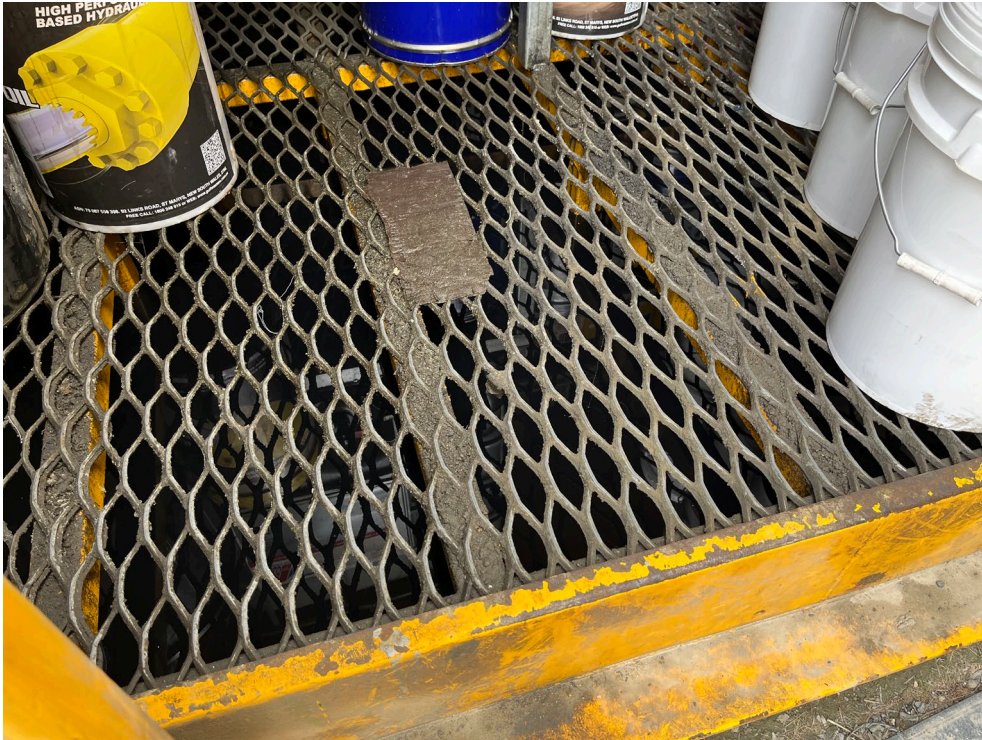
PHOTO 5 Hazardous Substances bund full of oily water.
