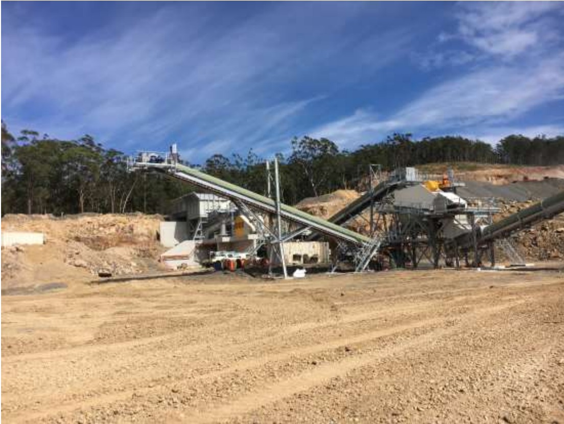
Plant completed. Extraction area shown in background. Photo taken.1 November 2017
